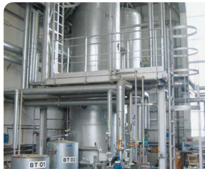
Glycol recycling facility at Munich airport.
